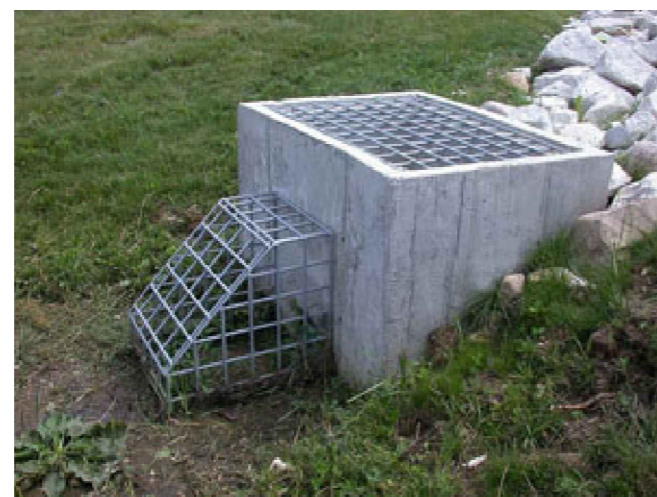
PHOTO OF SEDIMENT FOREBAY WITH RISER OUTLET (Alternative options corrugated pipe and concrete chamber)
