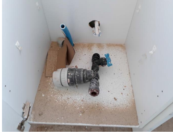
Internal meter install poor practice
